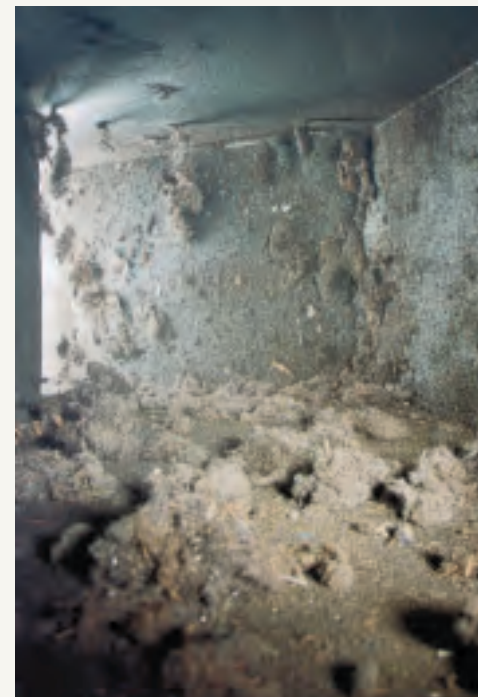
Dirty Duct: Accumulations of dust and debris within HVAC ductwork can contribute airborne particulate within a home or commercial building, while also reducing air flow and increasing energy consumption and related costs.
