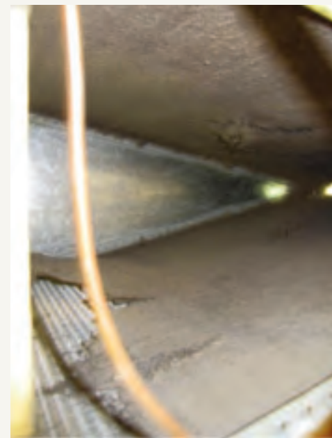
Fouled Coil: This photo shows the upstream side of a heavily-fouled A-coil, which is essentially matted over with dust and other contaminants.
