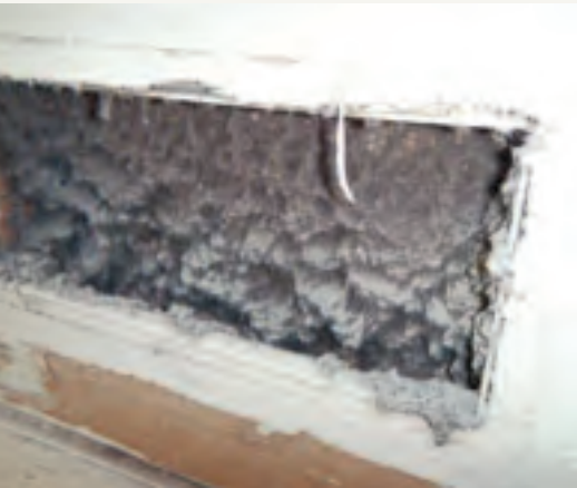
Clogged Duct: In extreme cases such as this, ductwork can become totally clogged, totally restricting air flow.
